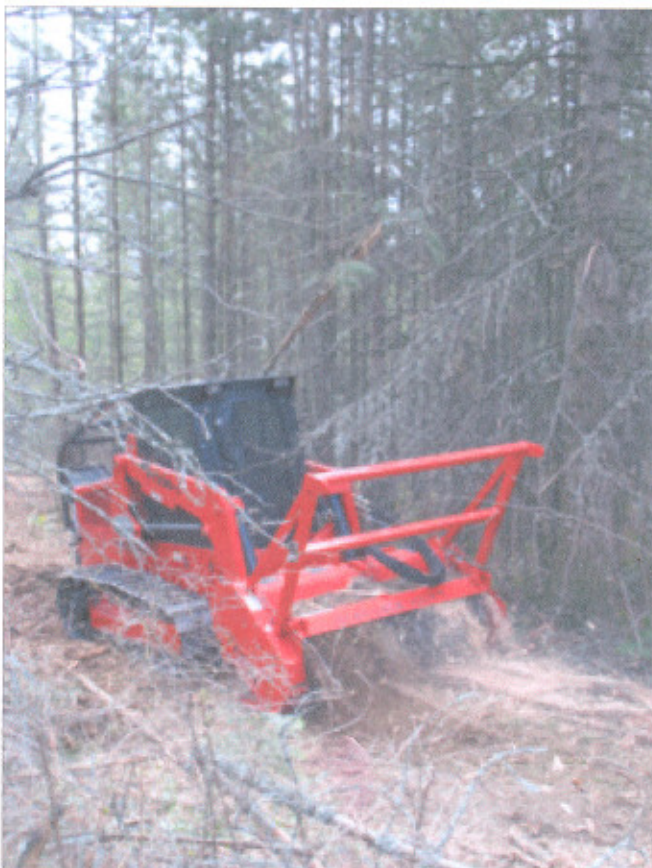
A Fecon FTX90 mulcher shreds underbrush and standing trees to six in. in diameter, making quick work of trail grooming projects.
